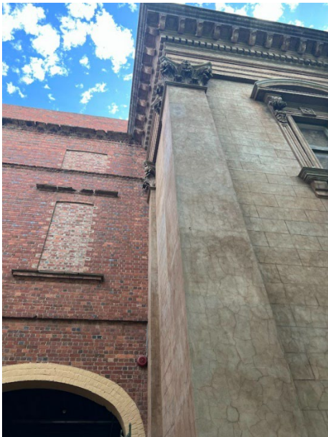
2023. Interface between original building and 1890 extension. 1890 extension was never rendered.
