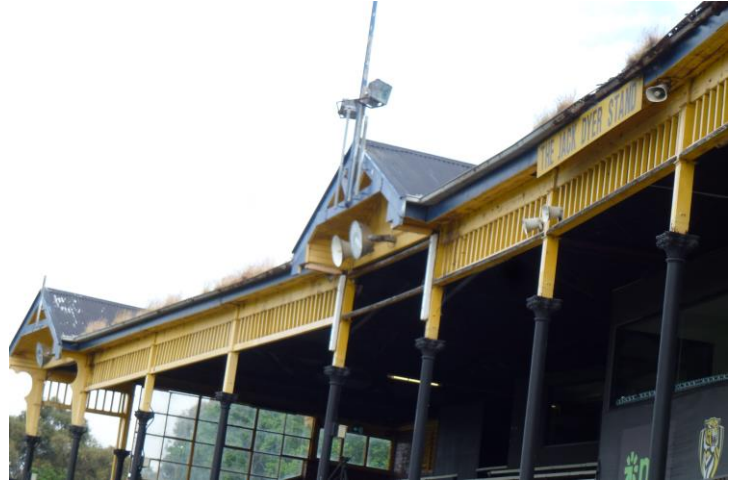
2022, Blocked and corroding gutters
