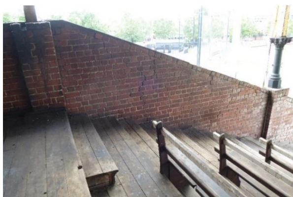
2022, Minor fire damage and cracks in brickwork
