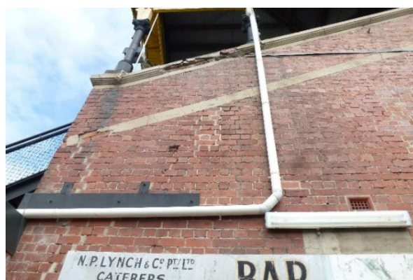
2022, Surface damage to masonry
