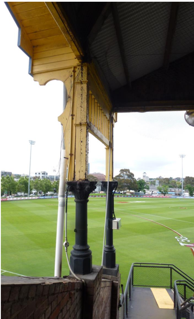
2022, Minor corrosion of iron uprights and new PVC pipe
