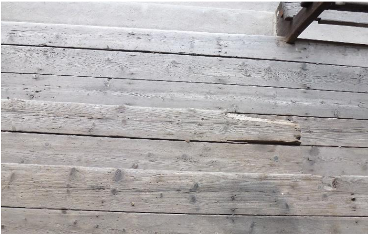
2022, Wear on floors
