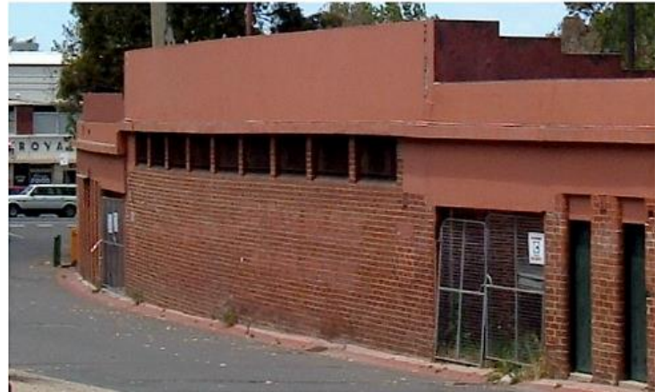
Undated, 1930s toilet block, most demolished before 1995. Source: The Holy Boots Football Emporium blog
