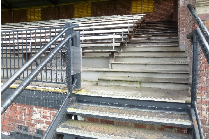
2022, White coating on stairs
